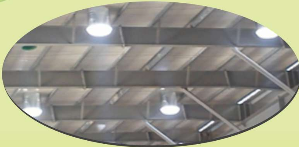
Pipe Cool Day Light system at MCF RBL
