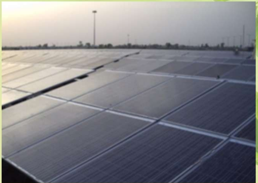
2 MW Solar PV plant at MCF RBL
